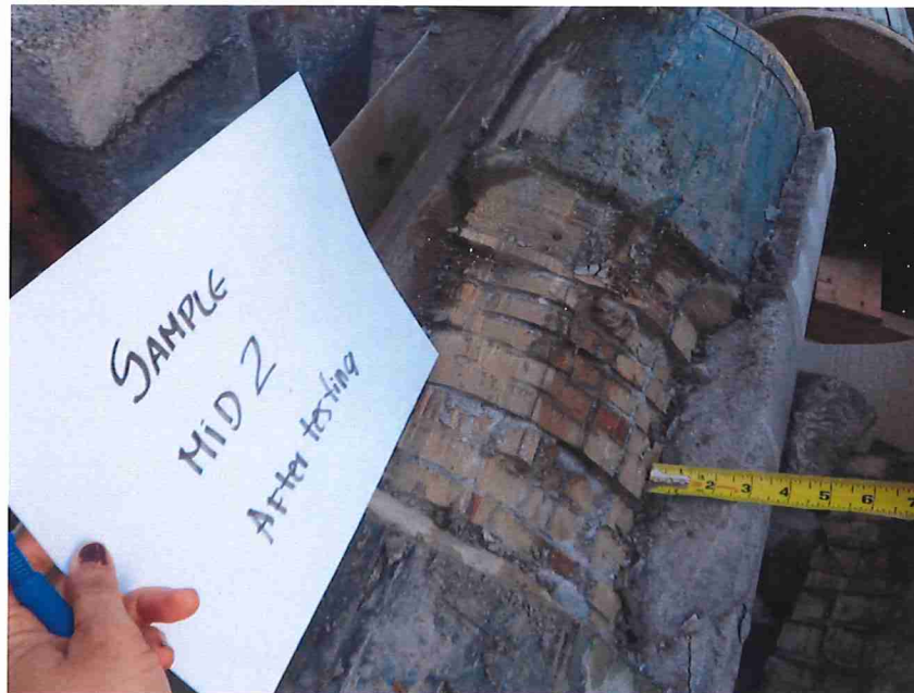
PHOTO NO.12 EXPOSING PILE REPAIRED AREA, NO WOOD DAMAGE IN REPAIRED SECTION OF PILE WAS OBSERVED
