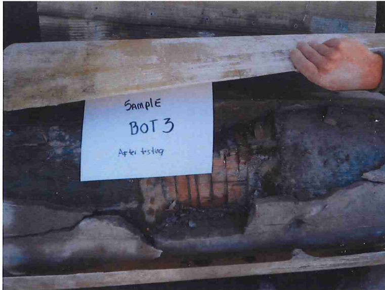
PHOTO No.10 EXPOSING PILE REPAIRED AREA, NO WOOD DAMAGE IN REPAIRED SECTION OF PILE WAS OBSERVED.
