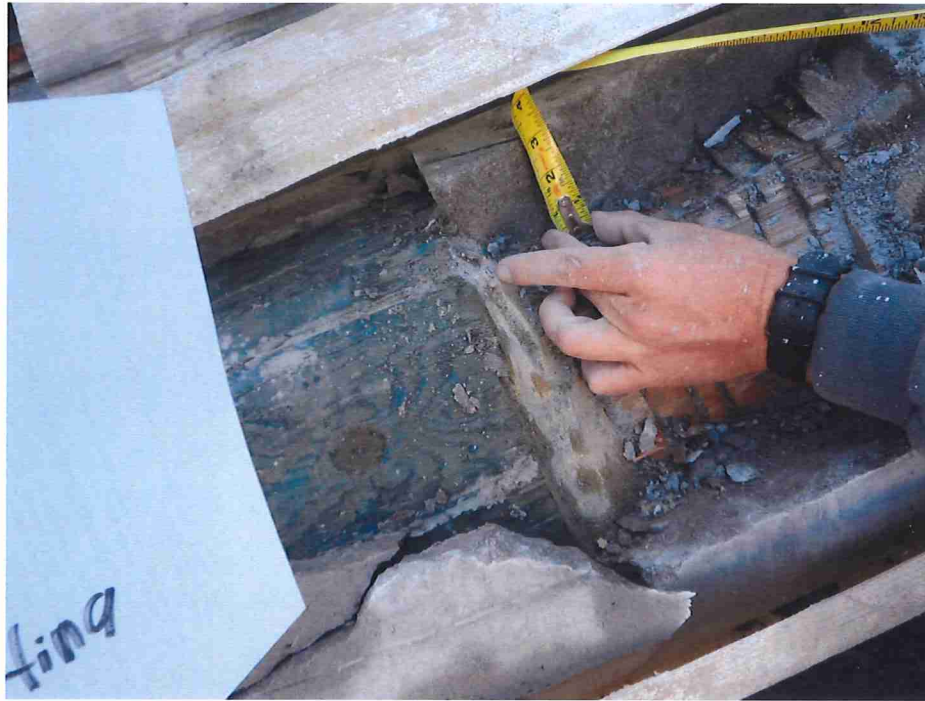
PHOTO NO.13 EXPOSING PILE REPAIRED AREA (MID 2 SAMPLE) , NO WOOD DAMAGE IN REPAIRED SECTION OF PILE WAS OBSERVED.
